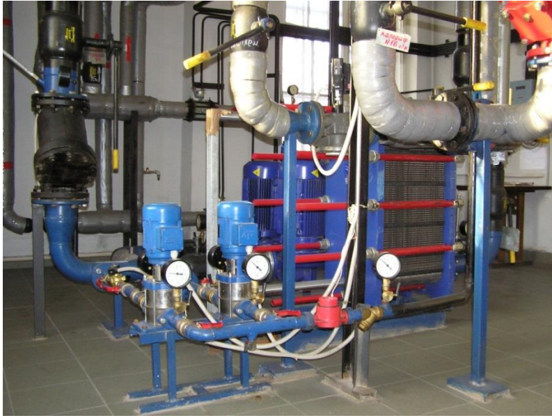
Figure 2. Individual Heat Substation with total capacity 1.2 MW in apartment building at Dnepropetrovsk produced and installed by SODRU.
