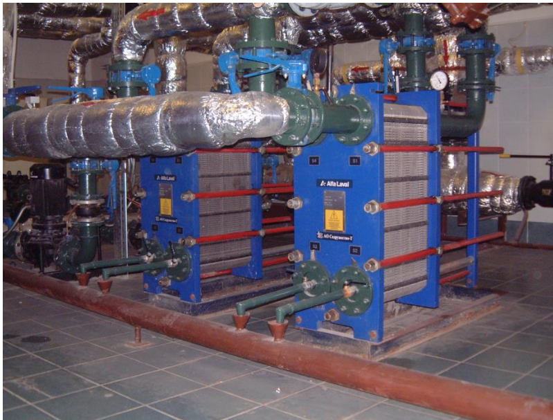
Figure 1. Central Heating Station with total capacity 10 MW at railway terminal in Kiev produced and installed by SODRU
